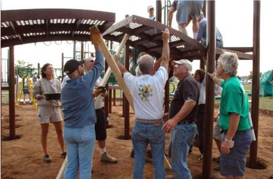
Neenah Rotary helps build another playground. Rotary members have become experienced playground builders after completing projects at Washington, Green, Great Northern, Riverside, and now Memorial parks.
